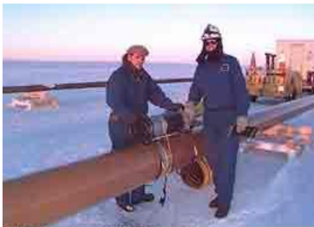
Photo Courtesy of Yxlon International
